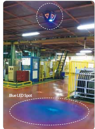
▶ Factory Indoor / Crossway ZT
